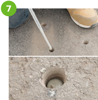
Insert nozzle and fill each hole to 1" below floor level with adhesive.
